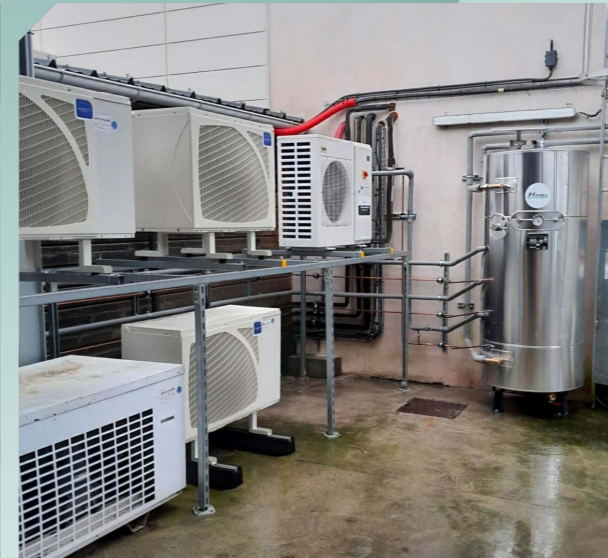
Station service - 500 L
